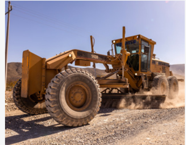
RURAL ROAD MAINTENANCE AROUND LA ENCANTADA MINE
