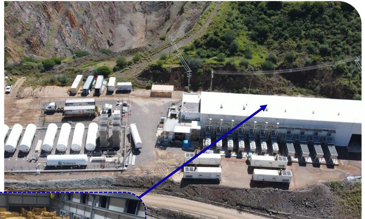
Santa Elena's 24MW LNG Power Plant
